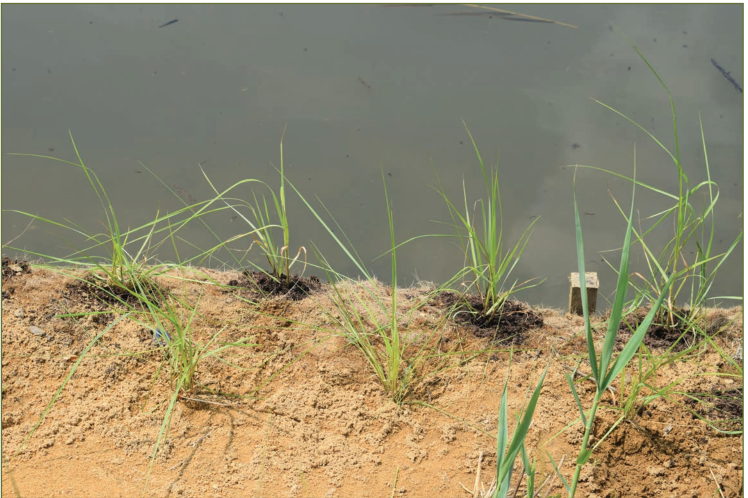
600 plugs of Spartina alterniflora were planted into the coir logs and backfill.
